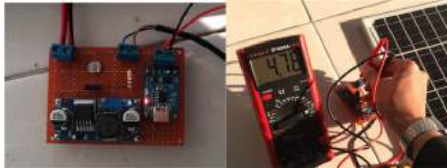
Figure 4. Maintenance Solar Panel System
