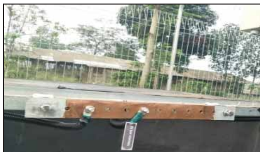
Gambar 4. External grounding box
