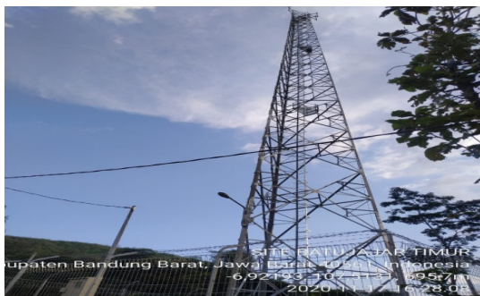
Gambar 1 Menara BTS ( Base Transceiver Station )
