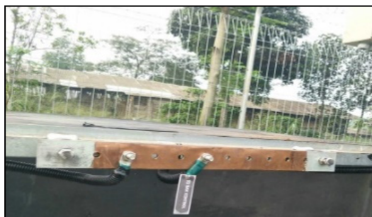
Gambar 4. External grounding box
